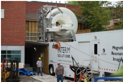
MRI Magnet Removal: Old magnet is lifted by crane from Oakville-Trafalgar Memorial Hospital's entrance to a flatbed truck and removed from site.
