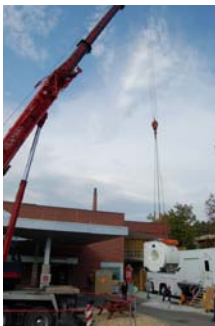
New MRI Magnet Delivery: New MRI is lifted from flatbed truck to hospital's entrance and transported to the MRI Suite for installation.
